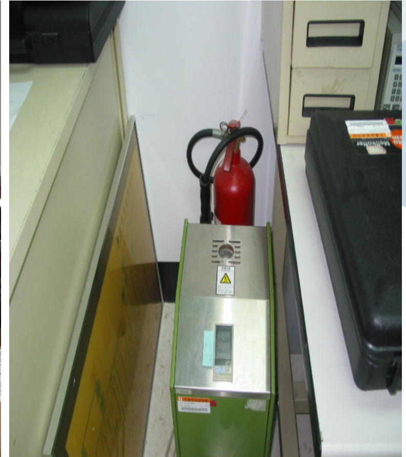
Fire extinguisher obstructed by instruments
