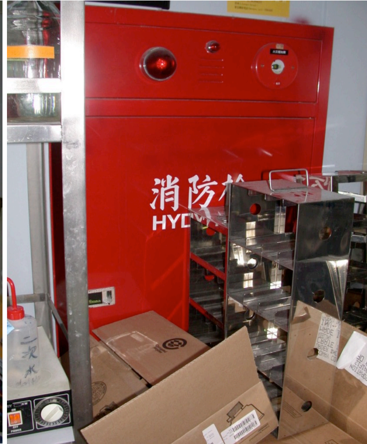
Fire hydrant obstructed by Furniture, Cardboxes
